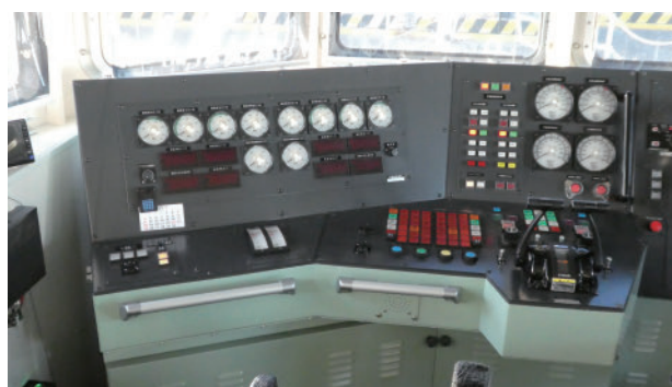
Photo 12. Bridge console for engine
