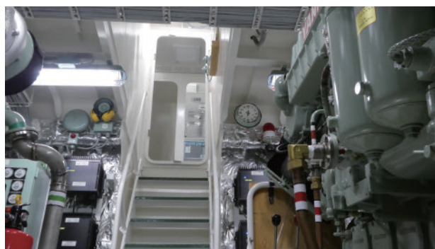
Photo 11. Engine room entrance
